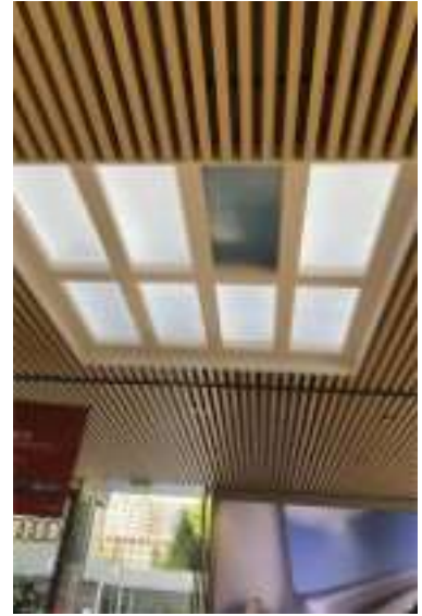
Single light not lit (not even dim)
