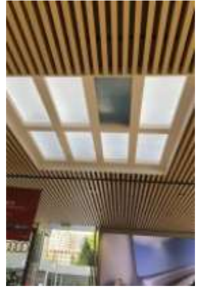
Single light not lit (not even dim)
